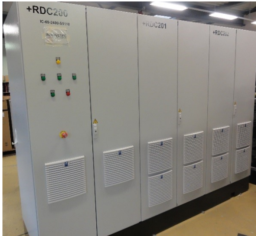
Picture 7: grid converter unit
