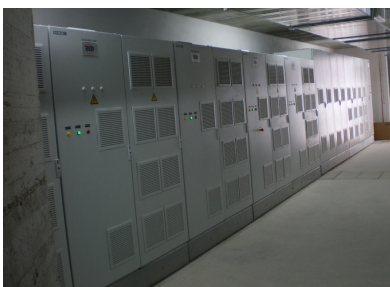
Picture 11: energy storage units
